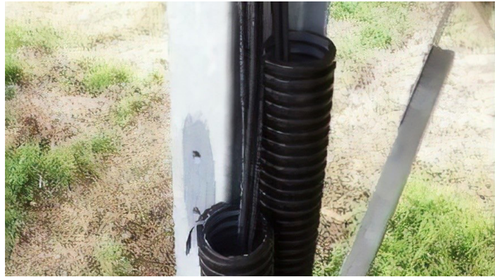
Figure 8: Unsealed cable ducting
