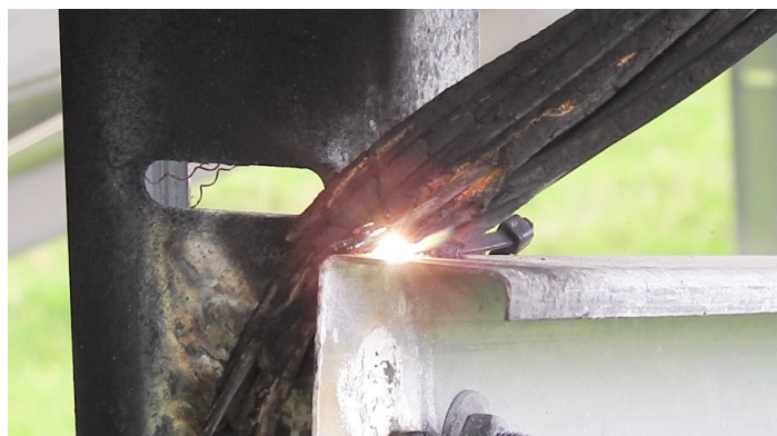
Figure 10: DC string cables on fire
