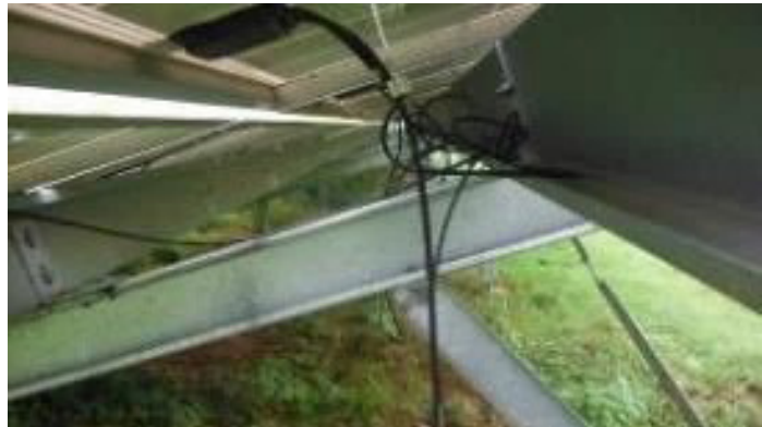
Figure 9: Inadequate cable management
