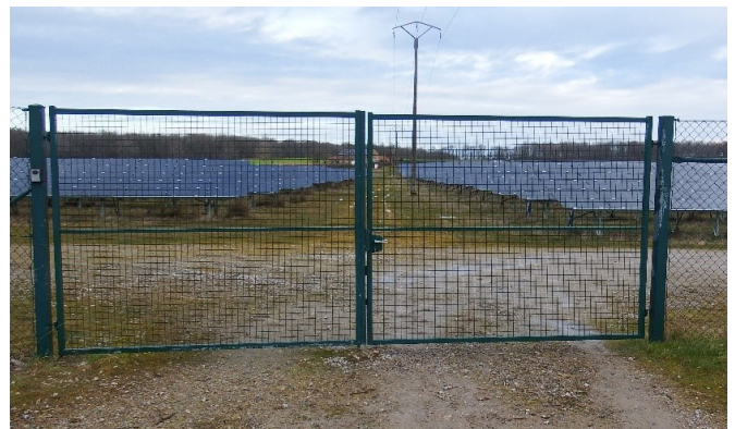
Figure 7: Missing identification on PV plant access gate
