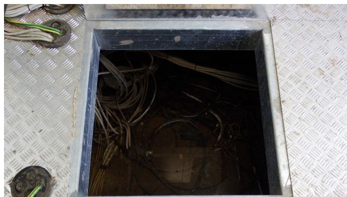
Figure 12: Water in substation foundations
