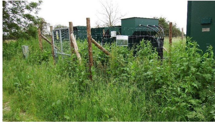
Figure 16: Grown vegetation around a substation
