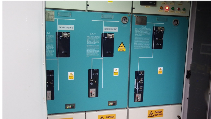
Figure 13: Missing locking mechanisms (padlocks) in switchgear cubicles
