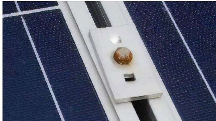
Figure 5: Module clamp corrosion on fixing
