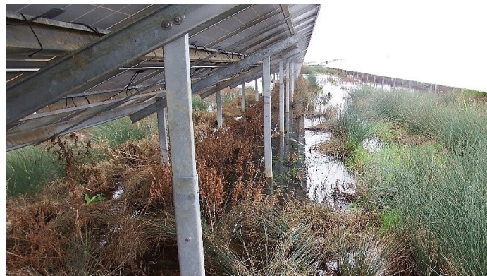
Figure 14: Waterlogged area in a PV plant
