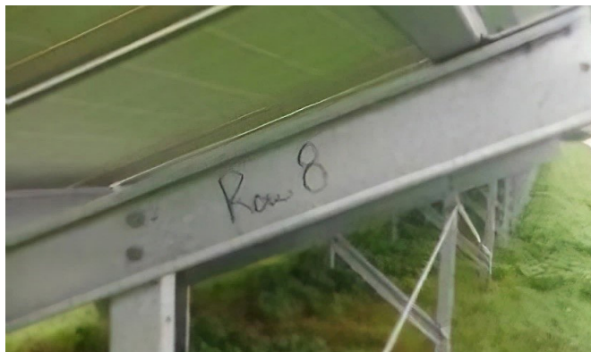
Figure 6: Inadequate identification of mounting structure row
